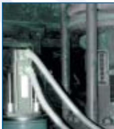
DEMC Linear Actuator Installed on a HP Hydraulic Servomotor of 300MW Utility Steam Turbine
