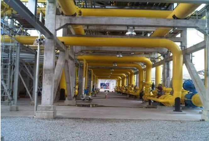
Fig.1 An Important step in preventive maintenance is monitoring ongoing machine operation and performance for irregularities. This includes monitoring the mechanical condition of rotating equipment and performing scheduled inspections of pipework, valves, pressure vessels and other components.
