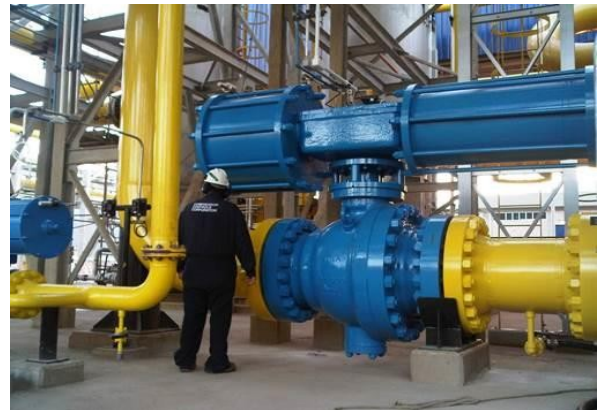
Fig.2 Regular audits by qualified personnel of suction and discharge pressures and temperatures, process gas flow rates, machine vibration, and steam flow, motor power, or turbine, power, can reveal significant details about a machine's health long before the overall process suffers.
